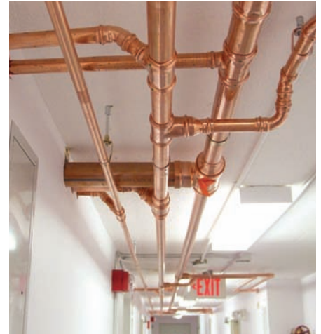
Exposed, press-fitted water service lines span the hallways of Kennedy Apartments in Concord, NH.
