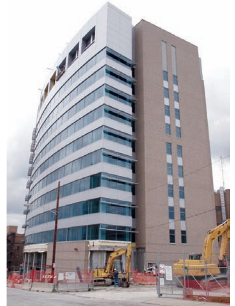
Children's Hospital Medical Center is building a new, 11-story research facility on its main campus in Cincinnati.
